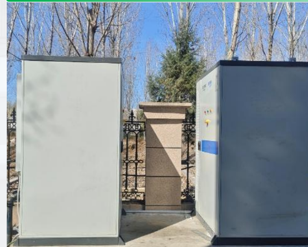
Tik Tok Data Center [2*96KWh] Commissioned in Jan.2025
