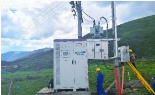
Distribution Energy Storage
