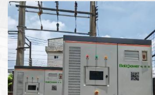
Transformer Capacity Expansion
