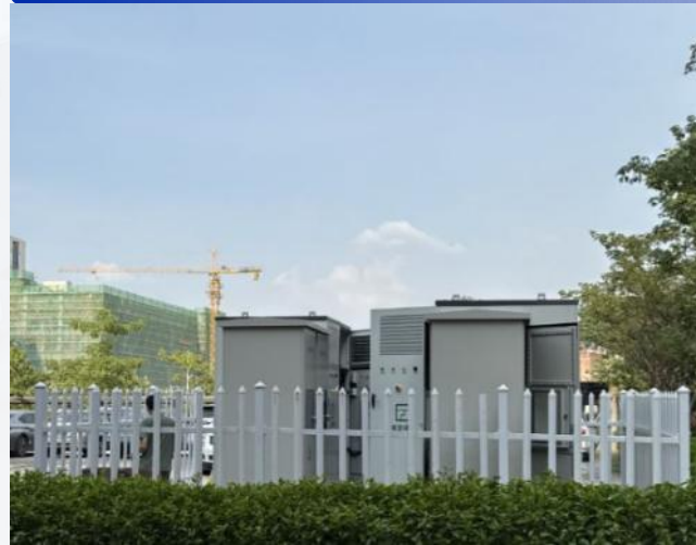
Guangdong [1.566MWh] Commissioned in Aug.2025
